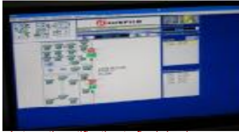
Automatic notification to fire brigade
